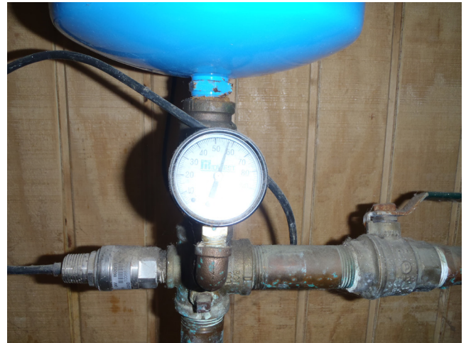
Figure 2. Pressure gauge on pressure tank.
