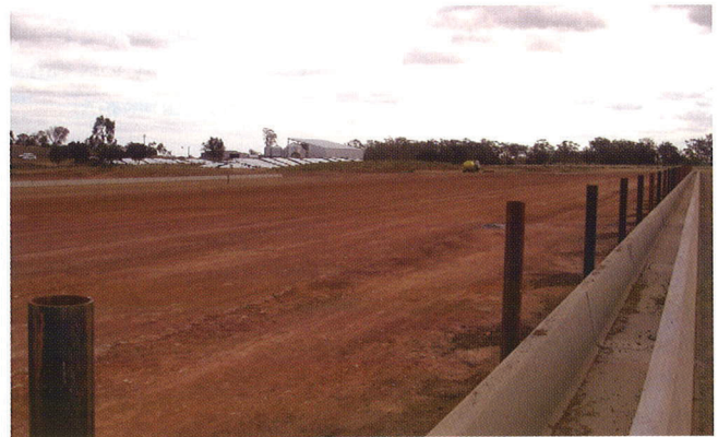
Figure 4. A pad or pen surface that has been properly graded and compacted before placement of apron and fence.
