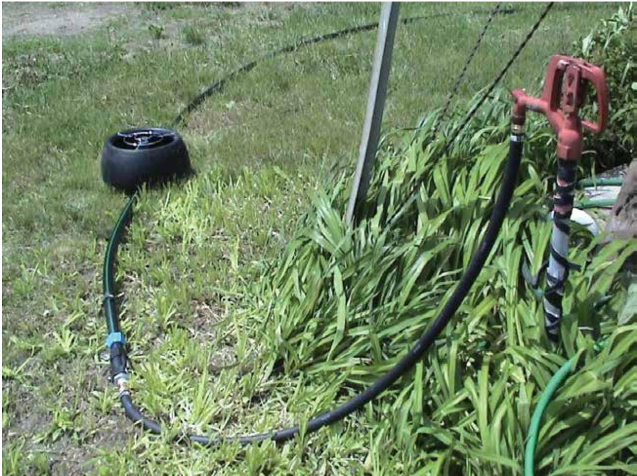
Figure 11. K-Line 1 1/4" tube connected to water hydrant with a Waterman AVP 1 air vent in the pod. Connections made using cam-lock fittings along the length of the tube. Photo credit Jason Gross.
