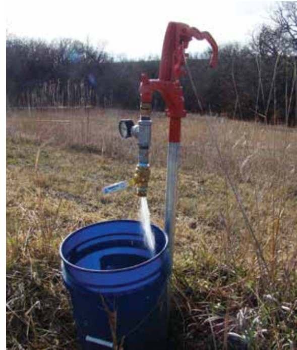
Figure 15. Assembly for measuring water pressure and flow rate from a hydrant. Photo credit Jason Gross.
