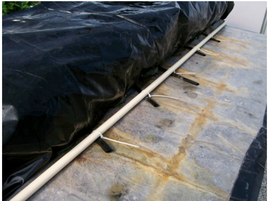
Figure 6. Ends of seep hoses are wire tied to 3/4-inch PVC pipe to maintain spacing between each length.
