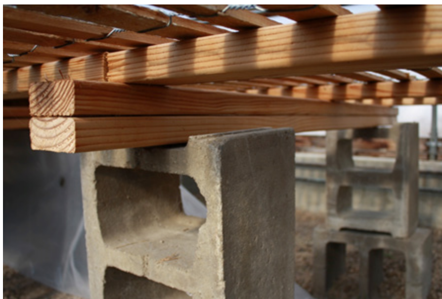
Figure 2. Cross-arm positioning with bench top support members and woven bench fabric installed.
