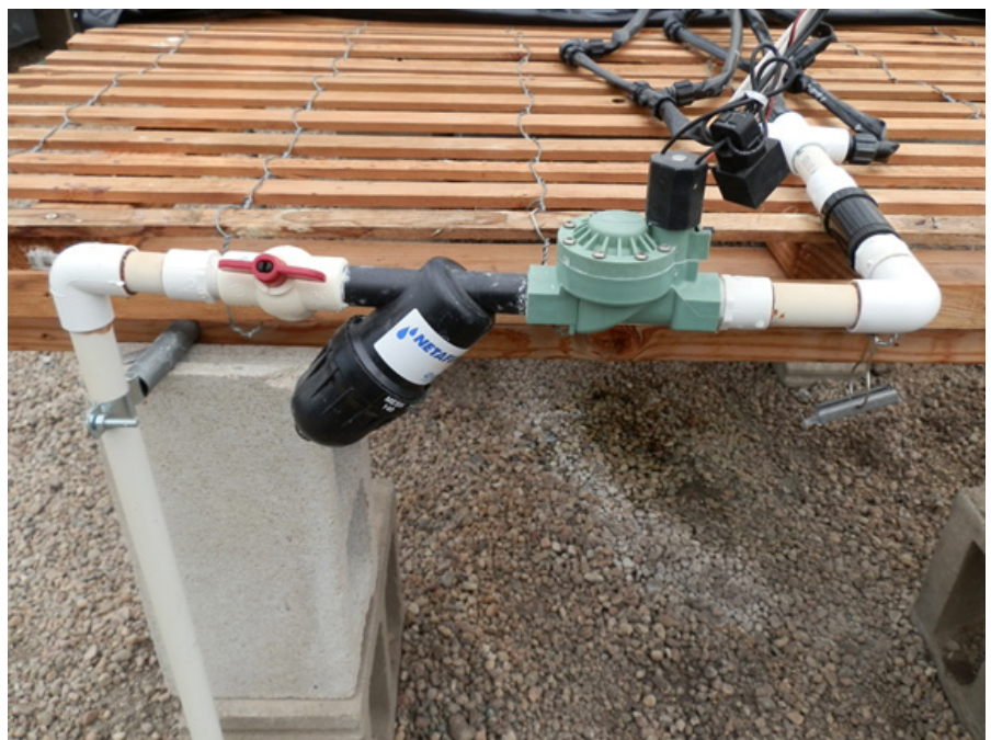
Figure 12. Irrigation supply to individual bench includes manual shut off, 140 micron mesh screen filter, 24 volt solenoid valve, and 10 psi pressure reduction valve prior to the Capmat II distribution manifold.
