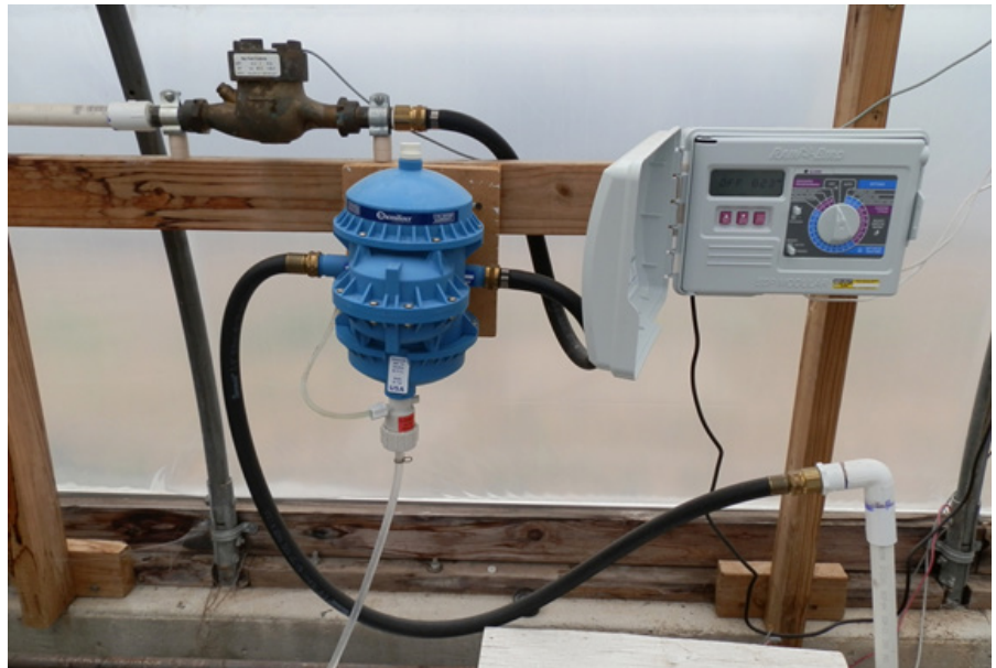
Figure 11. Irrigation supply line with water meter and fertilizer injector shown.
