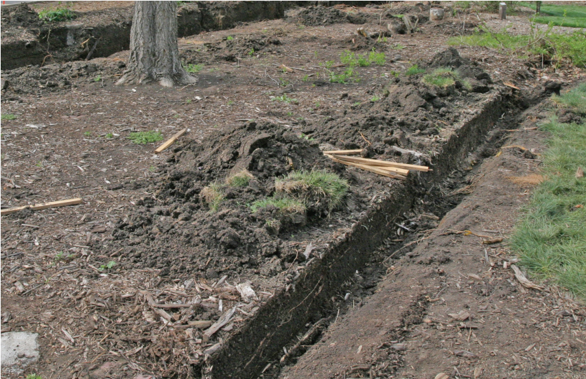
Figure 4. Existing trees also can be damaged by digging into their root systems to install new plants, or to modify utilities or irrigation systems. This damage can be minimized by designing the landscape to place plants at the outer edges of tree canopies, installing smaller plants, and hand-digging holes and trenches.
