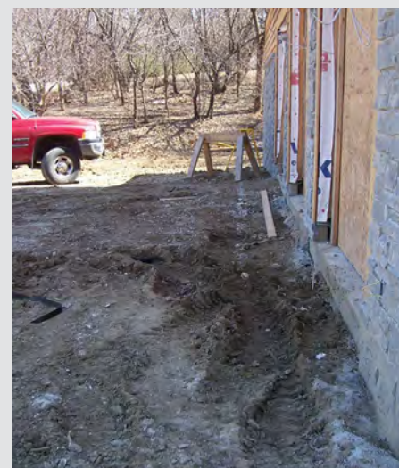
Typical home construction site with soil stripped of topsoil, putting the tighter, clayey subsoil, which is unsuitable for rain gardens, at the top.
